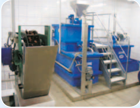
Chemical units – flocculant and coagulant
