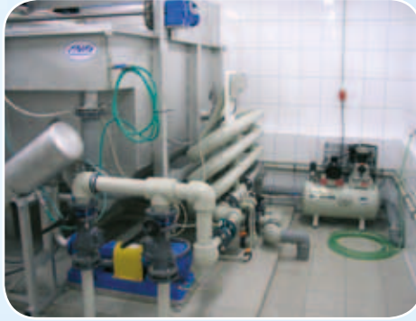
Pipe mixer next to flotation unit
